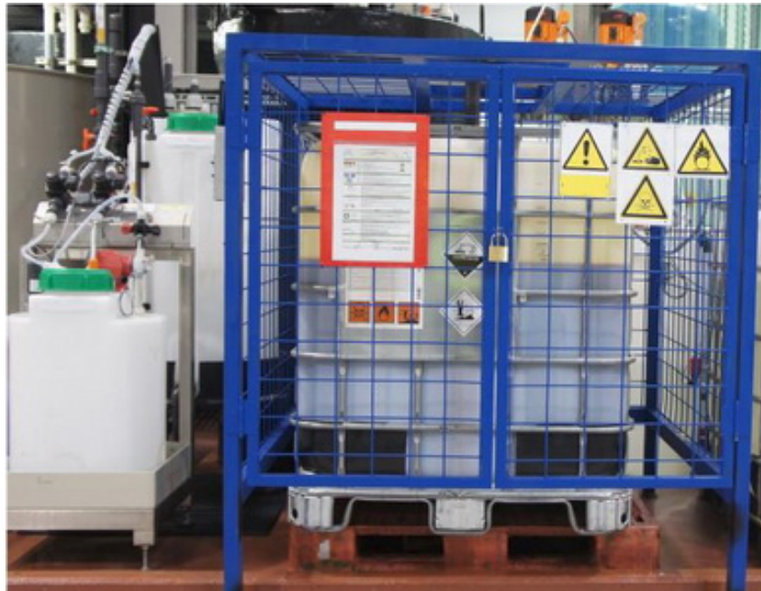
Figure 13 - Liquid hexavalent chromium additive pumping station.
