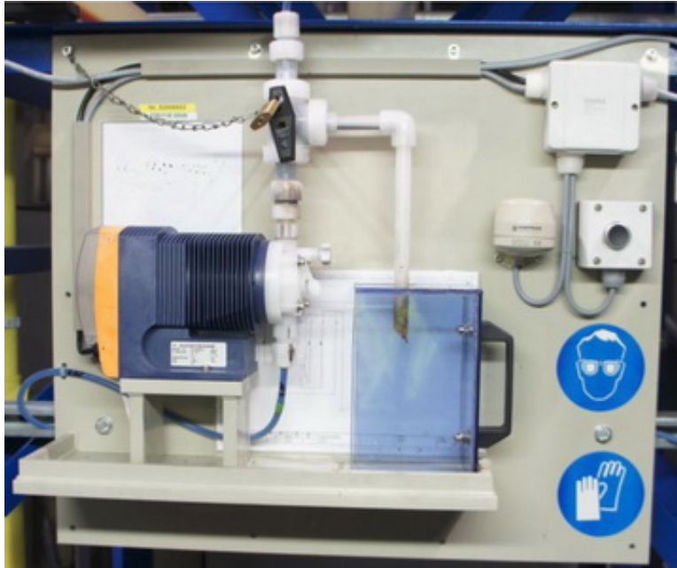
Figure 14 - Pumped sampling station.
