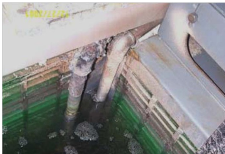
Figure 10 - Evidence of auxiliary equipment stray-current protocols being violated.
